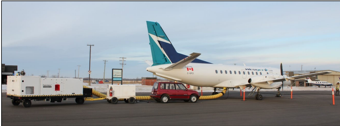
A Pre-Conditioned Air Unit (left) and Ground Power Unit (right)
